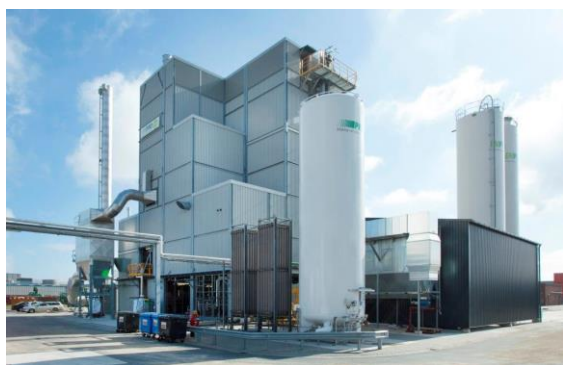
Figure 2: The Empyro demonstration plant
